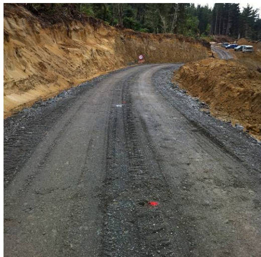
Figure 4: Once aggregate is applied over the geogrid the exact location is no longer visible.
