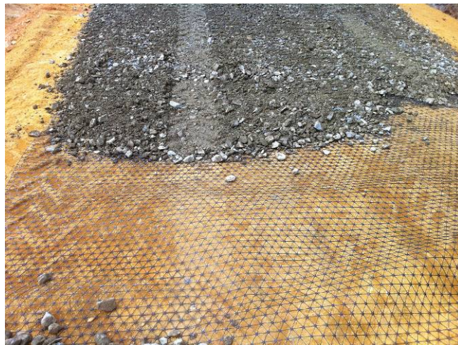
Figure 1: Geogrid, laid down on a forest road subgrade, being covered with a well graded aggregate.
