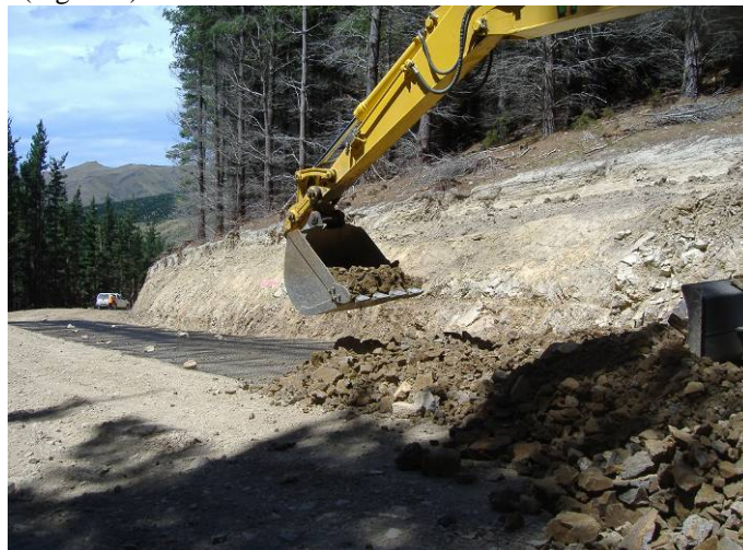
Figure 6: Spreading base course onto geogrid using an excavator. The maximum rock size in this aggregate is clearly too large and can easily cut the geogrid.
