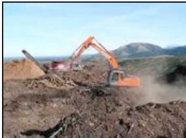
Figure 2. The excavator retrieving and piling the larger residue. The pile would then be hogged through the tub grinder.
