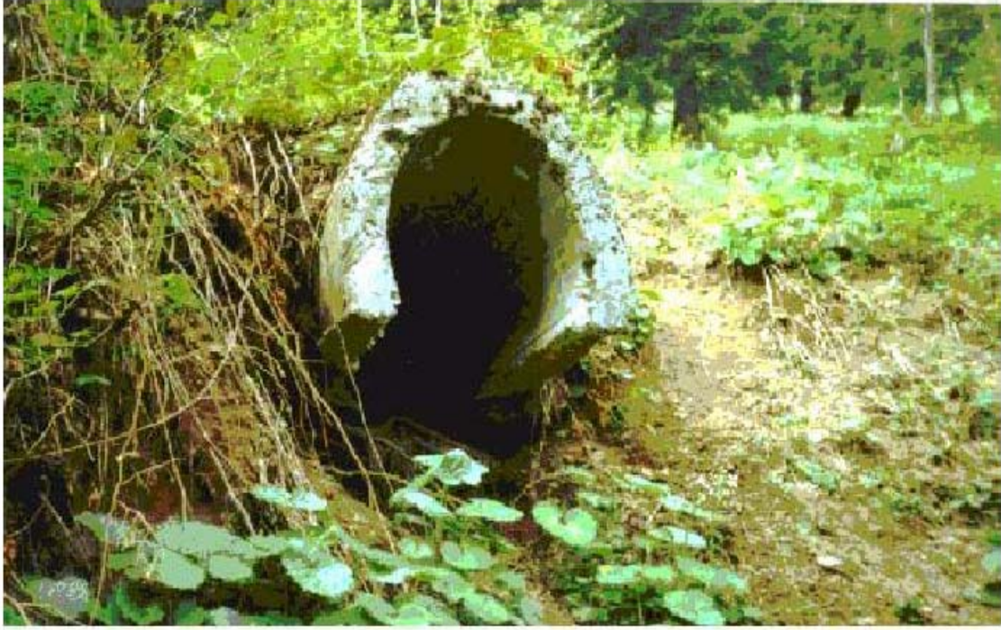
Figure 1: The destruction occurred on the end of a pipe due to improper building
